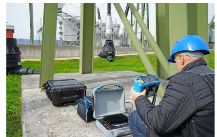
G-clamp reference point on the grid connection improving the result stability.
